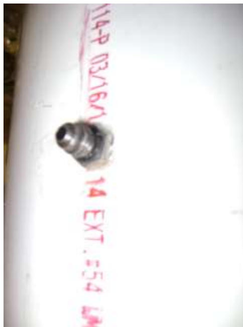
Figure 2 - Exterior View of Flare Fitting attached to Casing Wall
